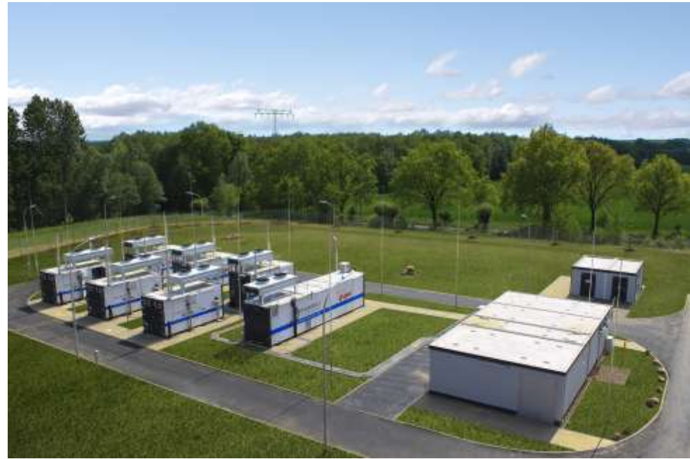
2MW Power-to-Gas Demonstration Plant in Falkenhagen, Germany
